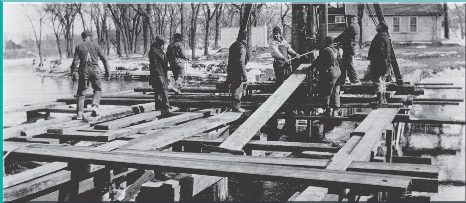
Figure 13. Employment on city public works projects, such as the construction on Fargo’s Fourth Street Dam in 1939, was usually limited to male heads of families. (Institute for Regional Studies, NDSU, Fargo, 2022.4.1)
